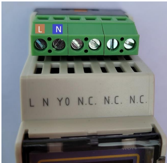
Top far left L = Live 240VAC Brown Wire Top left N = Neutral 0VAC Blue Wire
